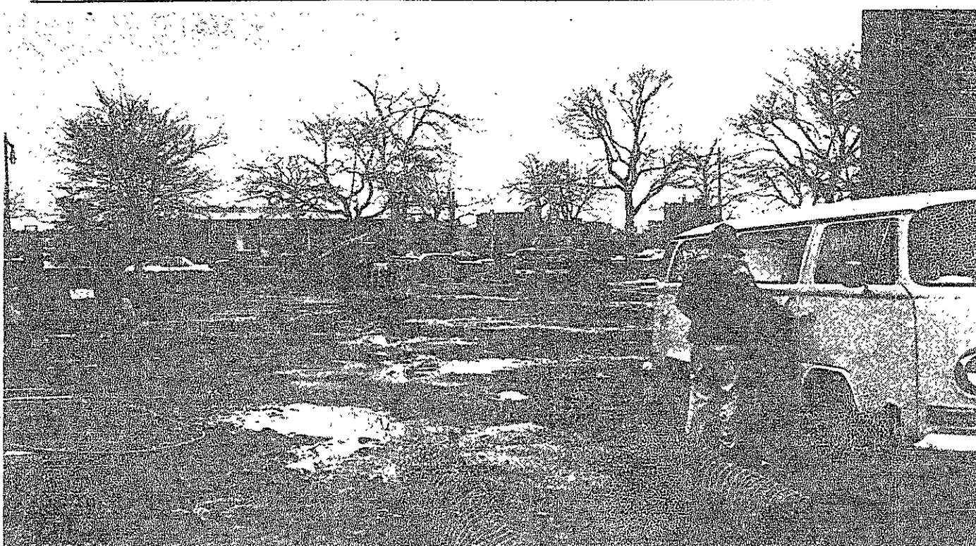
Construction began yesterday on the combined ATO and KS fraternity in the Burton Parking lot.
