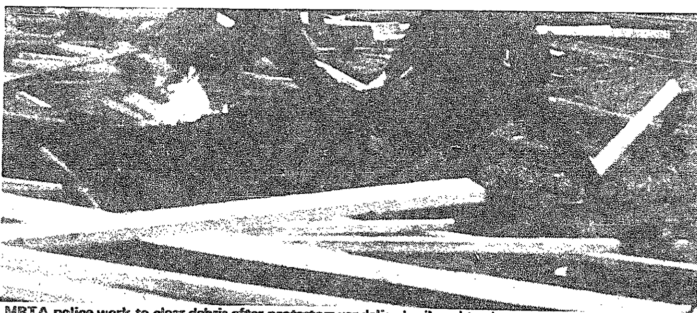
MBTA police work to clear debris after protestors vandalized railroad tracks. Photos by Dave Tenenbaum
