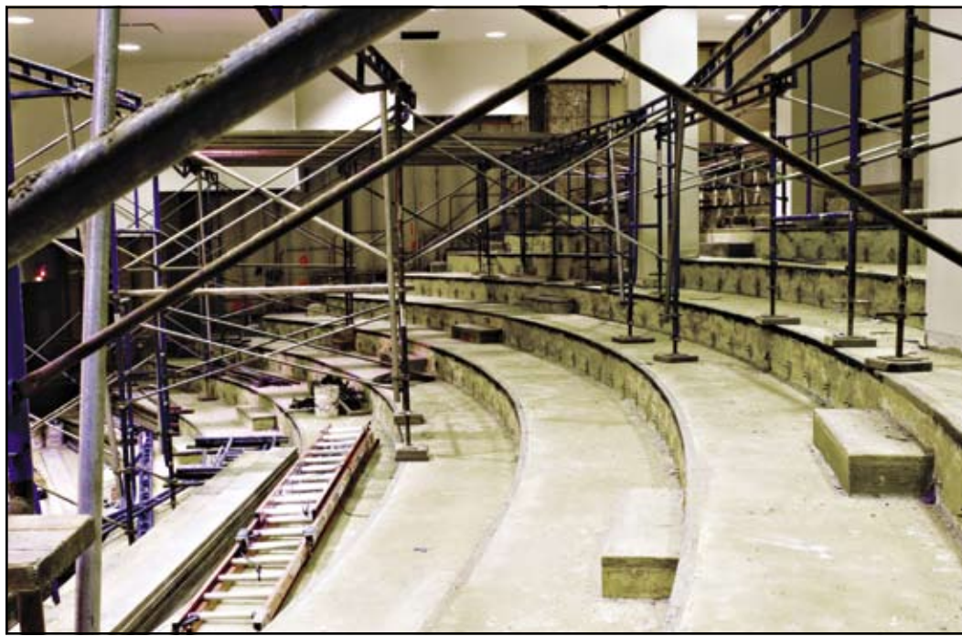
MIT's premiere lecture hall 10-250 is currently undergoing massive renovations, as seen on Sunday, Feb. 3. ERIC D. SCHMIEDL—THE TECH
