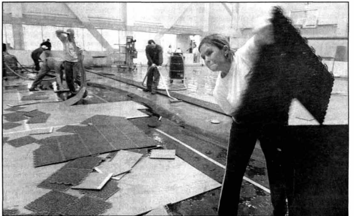
Workers remove the tiled surface of the 5,000-square foot Multi-Activity Court in the Zesiger Sports and Fitness Center Friday afternoon after a damaged fire sprinkler flooded the court. A repair time has yet to be determined.
