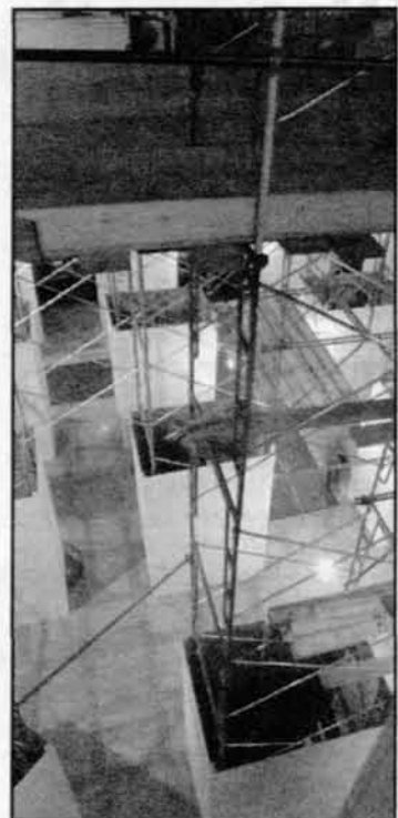
MATT T. YOURST—THE TECH Scaffolding was erected in Lobby 7 over spring break in preparation for major construction.
