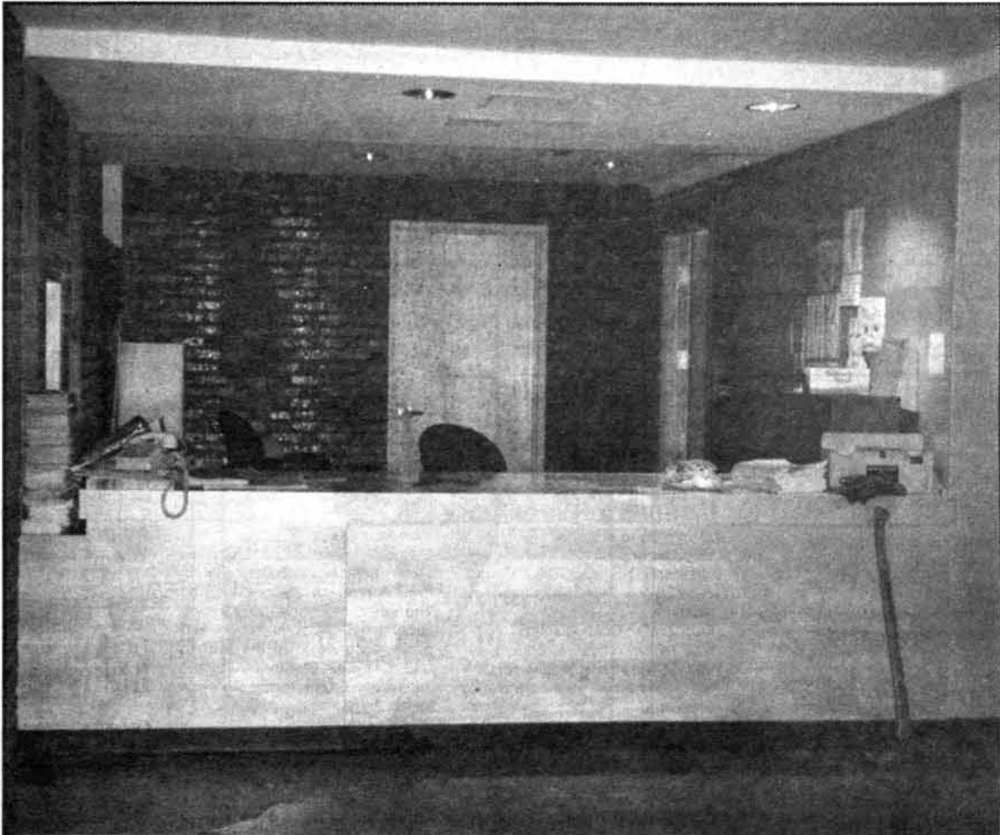
A freezing pipe triggered a fire sprinkler near Baker House's front desk Wednesday evening, causing a small flood.
