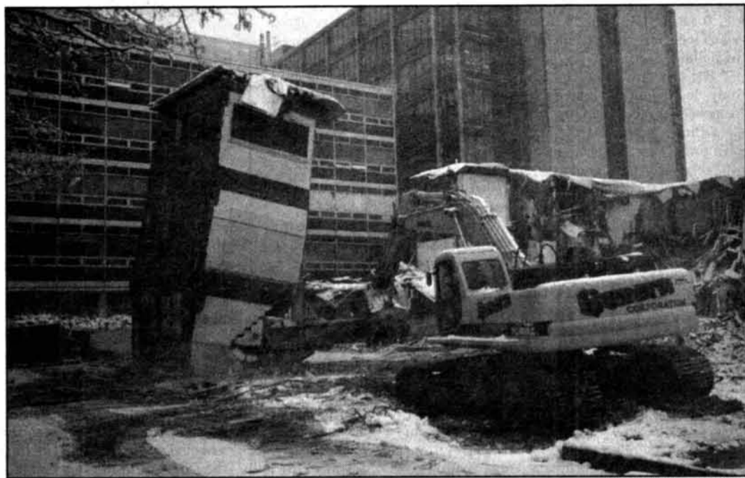
OUT WITH THE OLD, IN WITH THE NEW — Building 20 is withering away piece by piece to give way to the new Stata complex.
