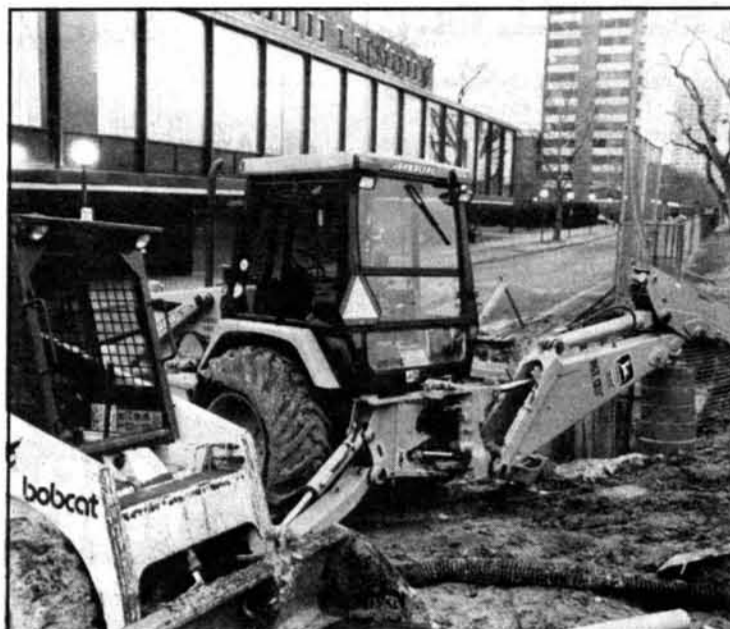
A bulldozer and backhoe parked at the construction site in front of Burton-Conner House.
