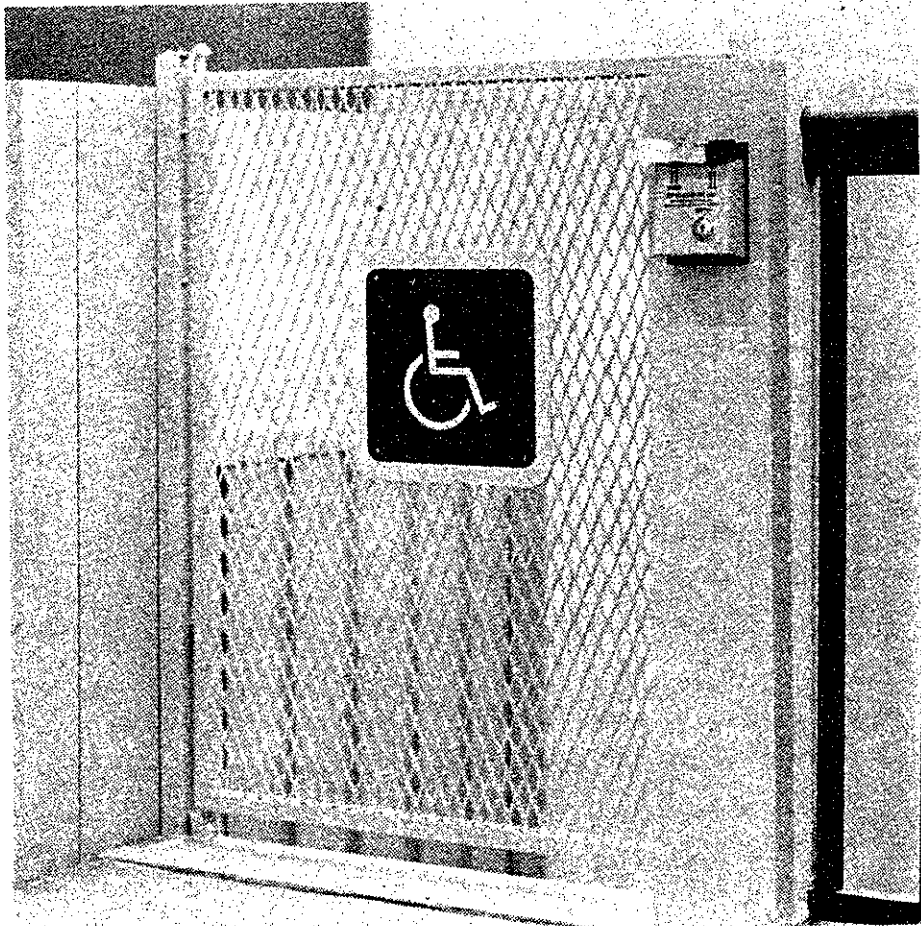
A wheelchair lift in Building 1 is part of MIT's handicapped accessibility project. (Photo by Steve Cohen)
